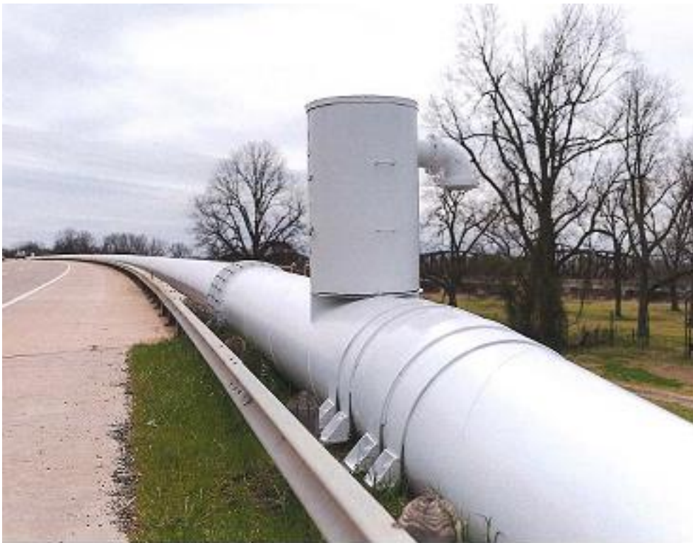
Painted Water Main
